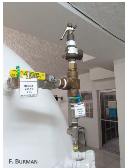
Dual safety valve
