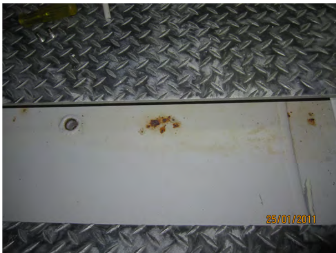
Reparable rust spots in the chamber bilge
